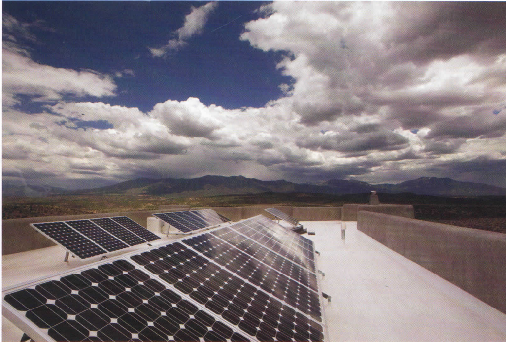
Solar panels on the roof provide enough energy for three to four days of power, and help shade the roof structure.
